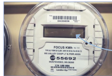
Digital meter: make sure this display is lit up.
